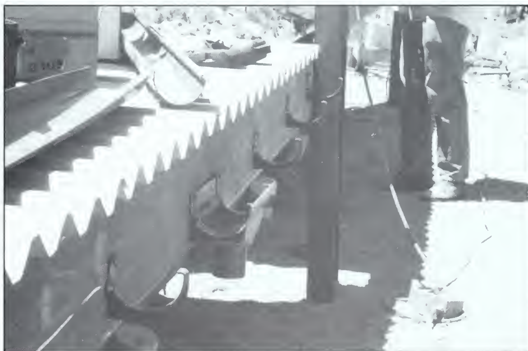
Photo 11. Guzzler gutter details: center drop and PVC gutter brackets are installed; pieces of the snap-in gutter lie on apron.
